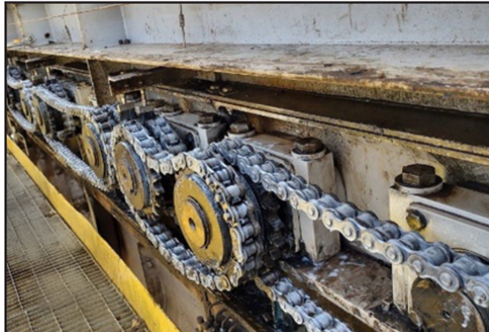
Log transport chains in woodyard experiencing excessive wear.
